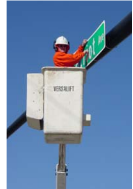
Public Works employee Bill Souder installs a new sign for Patriot Ave.
