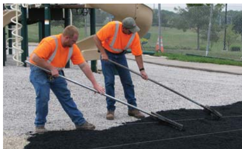
City Parks employees Mason Moore and Joe Loftin smooth out the crumb rubber surfacing.
